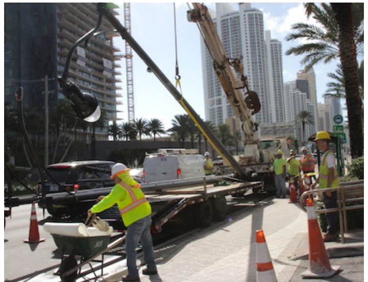
An undergrounding project takes shape in Sunny Isles Beach, Florida. Photo courtesy of the City of Sunny Isles Beach.
